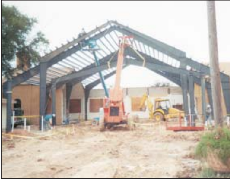
Skeletal steel frame expands the structure of St. Mary's building. (Photo by Gloria Johns.)
